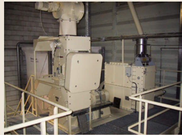
GLECHNER, PFARRKIRCHEN, GERMANY - VL3 ATEX HAMMER MILL DESIGN (ENTRY INTO SERVICE 2003) - WOOD GRINDING: 3 T/H (8 MM FILTER) FOR PELLET PRODUCTION 99% < 4MM
